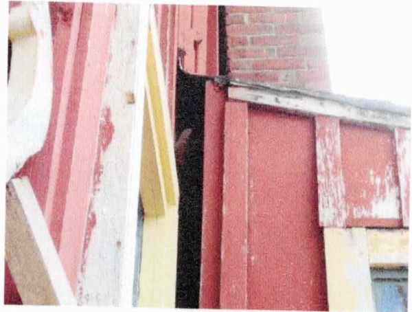
8) Exterior – North addition is separating from the main house; the chimney visible above the addition roof bears on combustible framing
