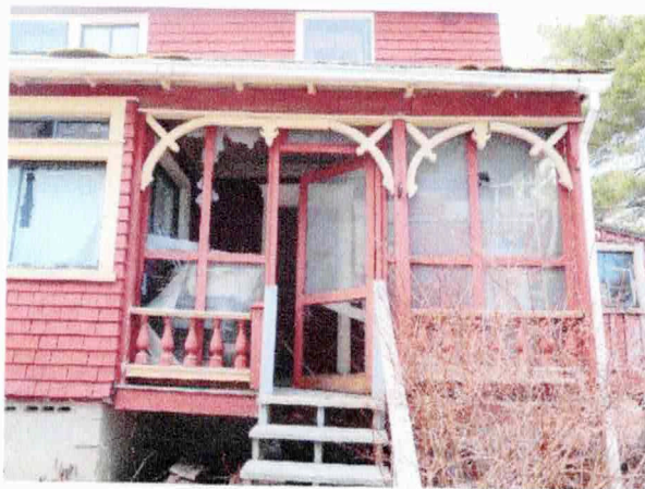
5) Exterior – Northeast porch roof and floor are structurally unsound
