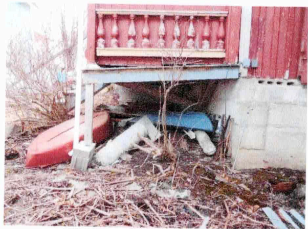
6) Exterior – Northeast corner of northeast porch lacks support; blocks are toppling over (not touching post); floor is deflecting downward
