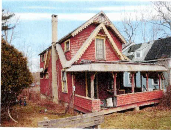
1) Exterior – South/west façades; south/front porch; porch has tarp roof; porch roof and floor are structurally unsound
