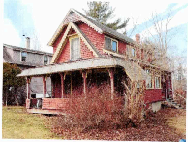
2) Exterior – South/east façades; south/front porch; extended overhanging entry porch roof is failing; porch is structurally unsound
