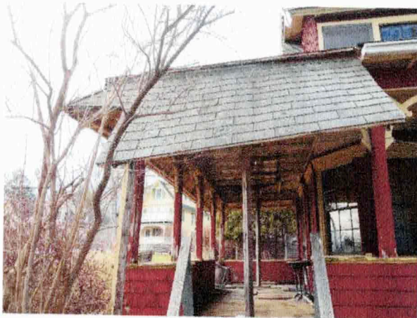
3) Exterior – South/front porch extended overhanging entry porch roof is failing
