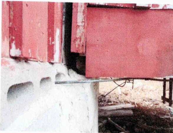
9) Exterior – North addition is separating from the main house
