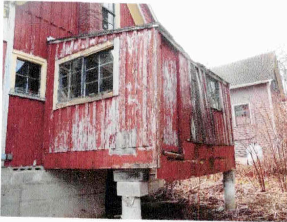
7) Exterior – North addition is degraded and appears structurally unsound
